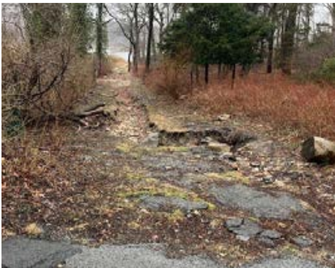
Erosion caused by stormwater runoff in the Hitherbrook Road area. Credit: Village of Head of the Harbor.
