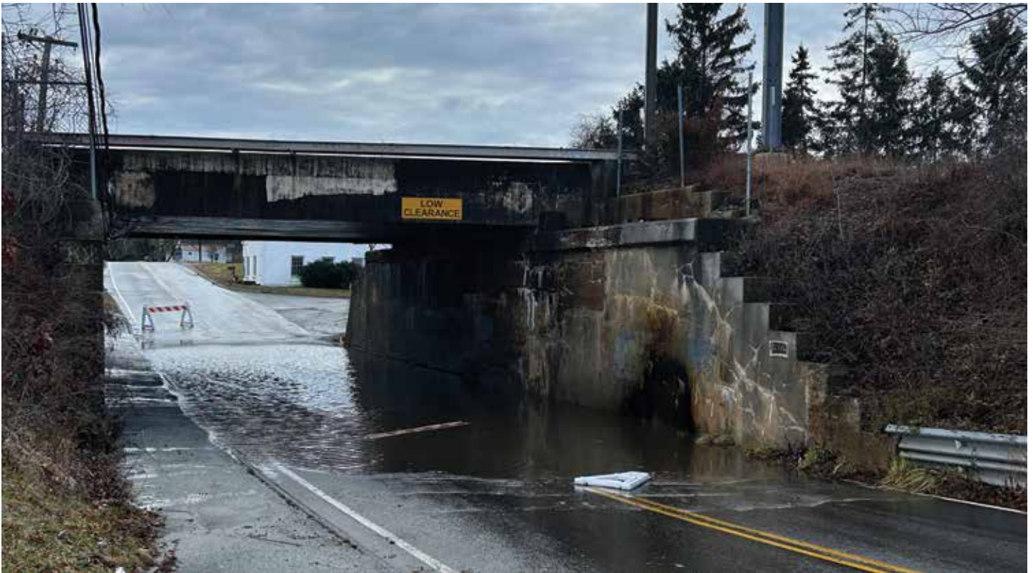
An underpass on South Road in Groton is flooded in 2024. Photo courtesy of Town of Groton
